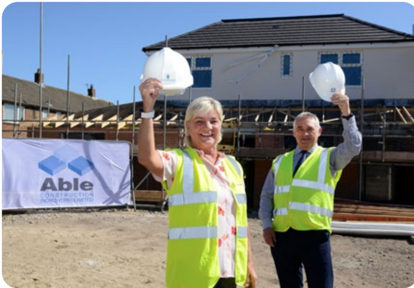
Cllr Liz McHugh with Able Construction Director Ken Parkin on the site of the new Children's Centre in Seton Avenue, South Shields.
