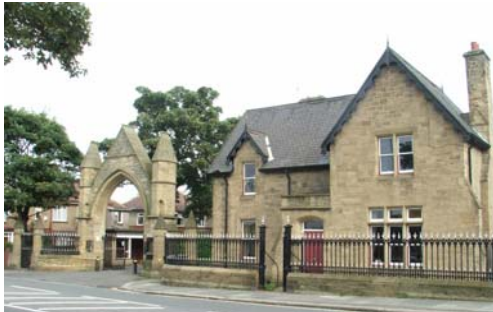
The Grade II Listed Cemetery Gates and Lodge are currently in good condition.
