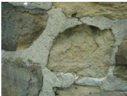
This wall has been re-pointed using a cement-based mortar. The softer stonework has eroded, leaving behind the hard mortar.
